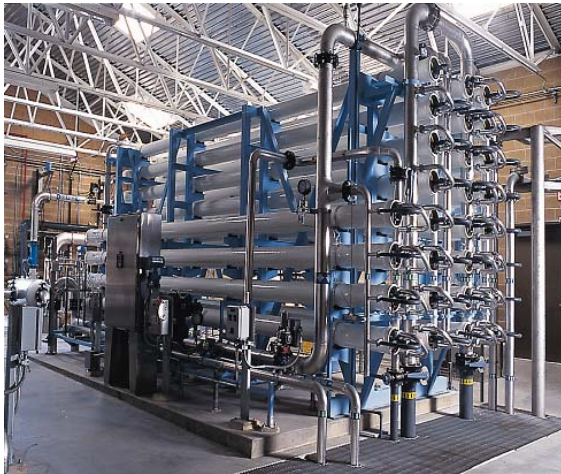
Figure 3.2. Membrane System Used as a Tertiary Treatment Process
